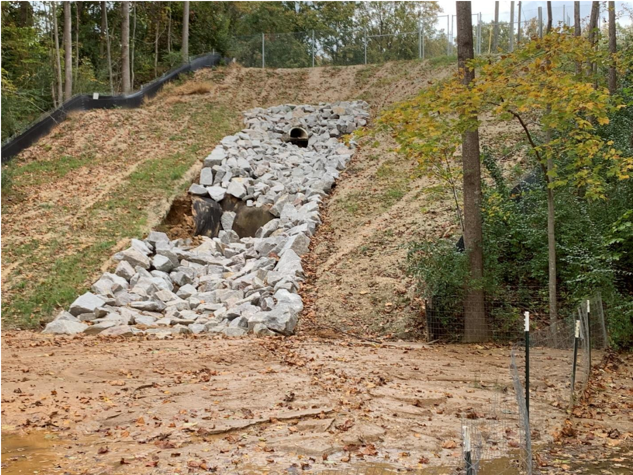
Discharging stormwater into an open channel on a steep slope seemed unwise from the beginning.
